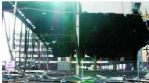
St. Thomas' Life Center was built in 2004. The building suffered severe damage during Katrina.
